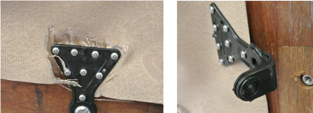
Figure 9: Tearing of fabric around a clip (left) and one clip pulled out (right) after Test 1
